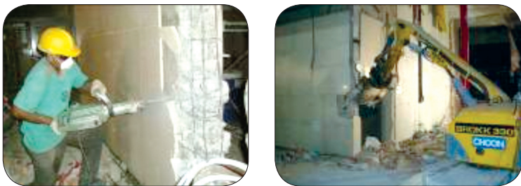
Figure 2: Substitution of jack hammer (left) with automated machine (right) to break concrete reduced the noise level from 90 dB(A) to 83 dB(A).
