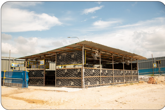
Figure 6: Shaded rest point for workers at a construction site equipped with rotating fans and water coolers. Encourage workers to sponge or rinse themselves with water e.g. during breaks. Body cooling is important especially on days when the weather is hot.
