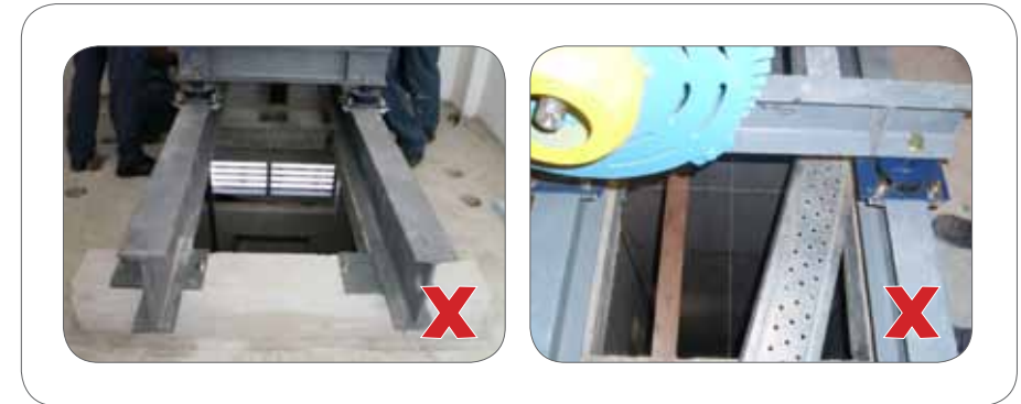
Figure 25: Falling through openings in machine room floor that were not properly covered during lift installation work.
