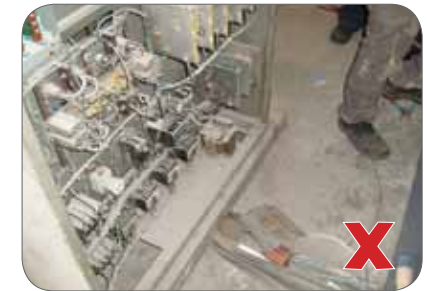
Figure 18: Worker can get electrocuted when he comes into contact with exposed electrical terminations.
