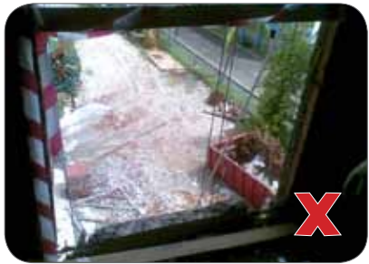
Figure 20: Falling off open sides at the roof or edges of buildings.
