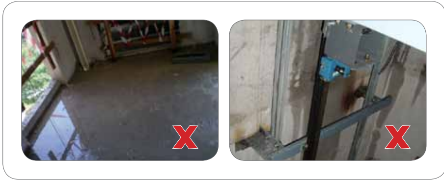
Figure 19: Worker can get electrocuted when he comes into contact with a flooded or damp hoist way.
