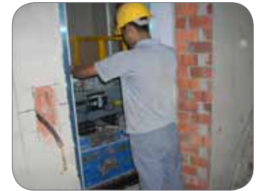
Figure 54: Proper checks must be done before accessing the car top.
