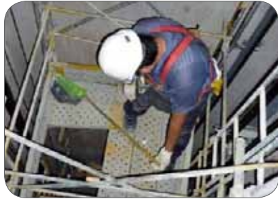
Figure 28: Falling off metal scaffolds.
