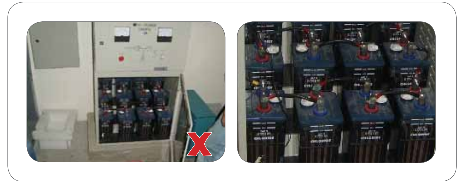
Figure 16: Electrocuted when worker comes into contact with improper insulated emergency battery operated power supply (EBOPS).
