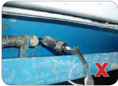
Figure 11: Damaged electrical cords.
