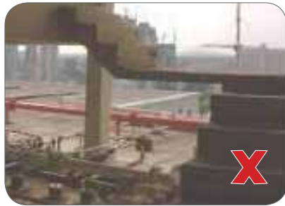
Figure 21: Falling off the unprotected edge of stairs.
