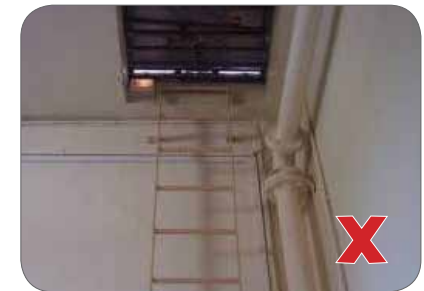
Figure 48: Example of cat ladder without hoops above 2 metres.
