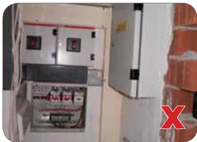
Figure 15: Wet or damp conditions due to water seepage into sub-controller.
