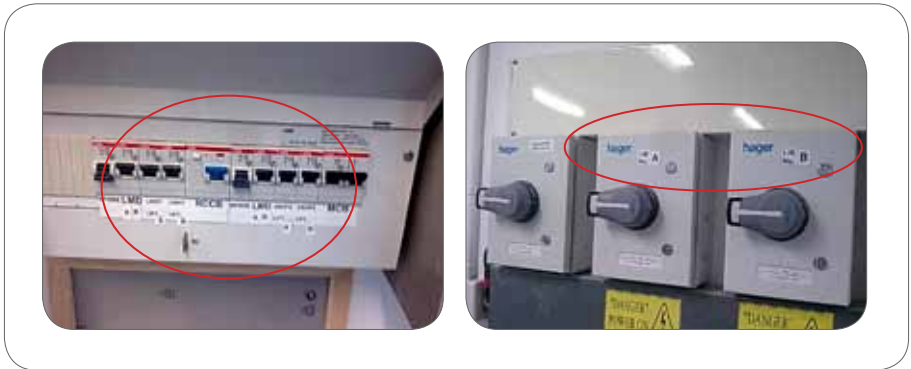
Figure 52: Examples of clear marking on lift isolators and distribution boards.
