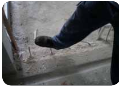
Figure 42: Slipping, tripping and falling due to uneven ground.
