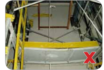
Figure 24: Falling off improperly constructed platforms and ladders when worker is using them to help replace ropes, sheaves, and so on.
