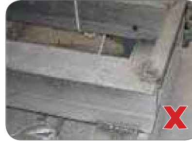
Sharp corners (cutting hazards).
