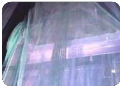
Figure 37: Netting partition used to isolate hoist way to prevent workers from being hit by items accidentally dropped from other hoistways.
