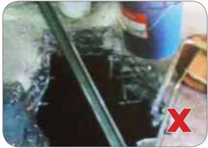
Figure 29: Potential fall hazard—floor openings in motor room.
