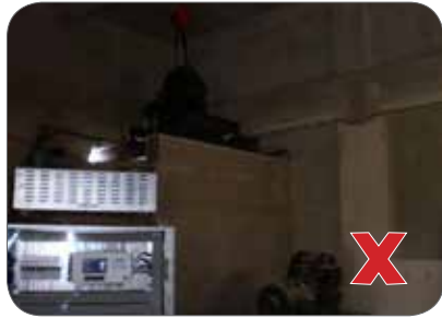
Figure 30: Falling off elevated secondary machine rooms with no railings.
