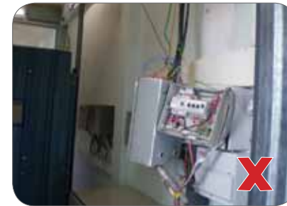
Figure 17: Worker can get electrocuted when he comes into contact with defective electrical equipment.
