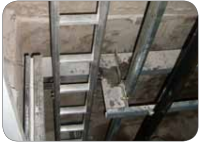
Figure 31: Falling off pit ladders.
