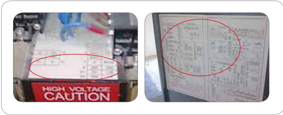
Figure 51: Examples of clear marking and labelling on electrical wires and terminal blocks.
