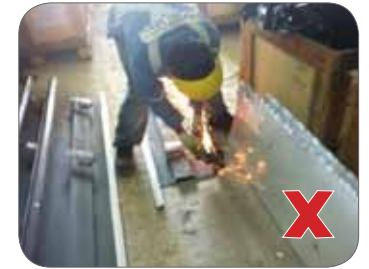
Figure 38: Fire hazard presented by welding, grinding, plasma cutting or gas cutting (above).
