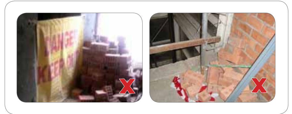
Figure 33: Equipment or materials falling through landing door into hoist way.
