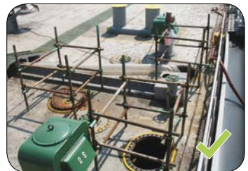
Guardrails for manhole openings.
