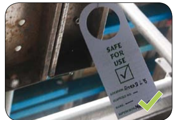
Equipment, such as scaffolds, need to be checked and approved before use.
