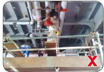
The worker is working on an inadequate working platform and the boards are not secured. He is also not wearing a safety harness.
