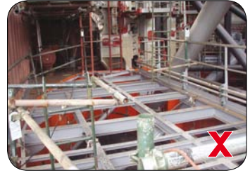
Steel erection may result in workers having to work on high, narrow working surfaces.
