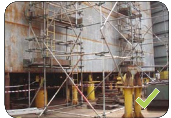
Proper means of access to scaffolds need to be provided.
