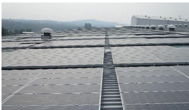
Sufficient space allocated for maintenance
