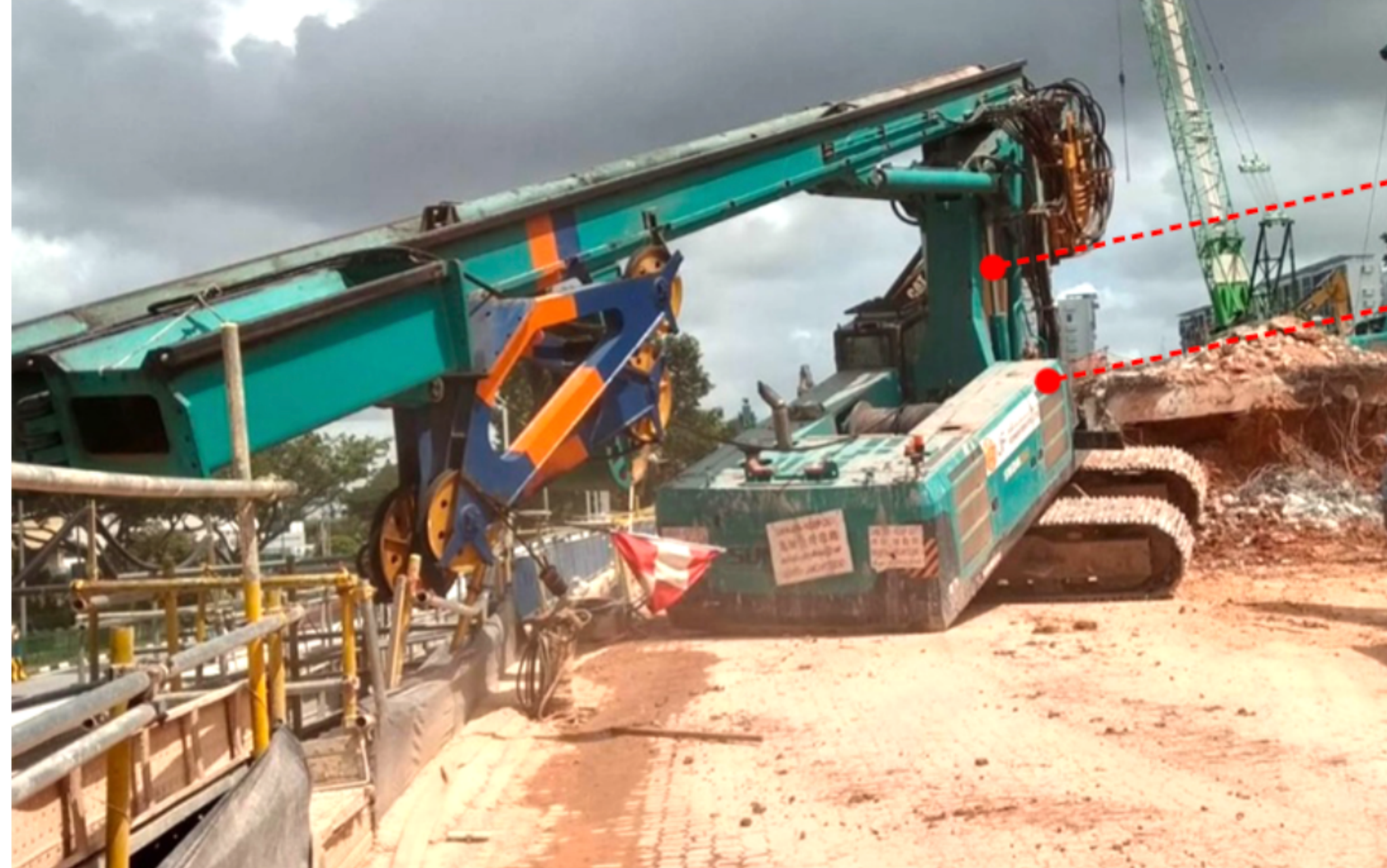
Overview of accident scene.
