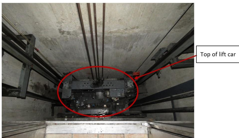
Figure 1: Scene of the accident.
