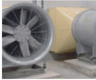
Exhaust (pull) ventilation for air extraction and enhanced air movement
