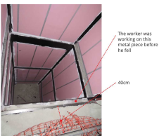
Figure 2: Distance from the guard rail to the open side of the lift shaft.
