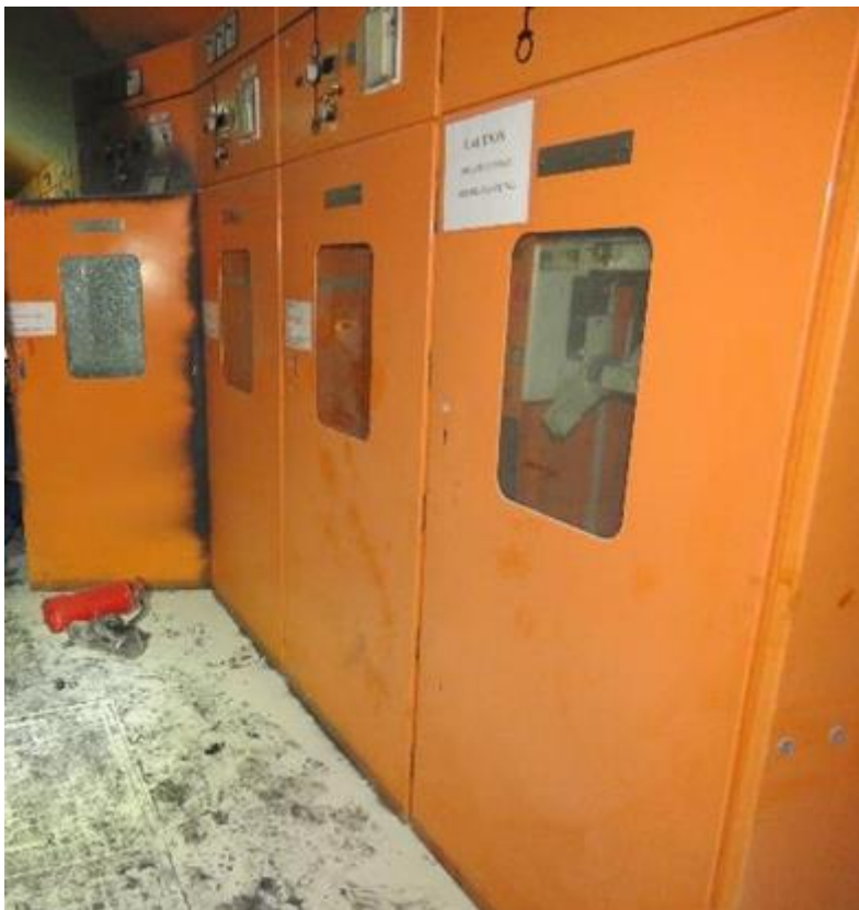
Overview of accident scene.
