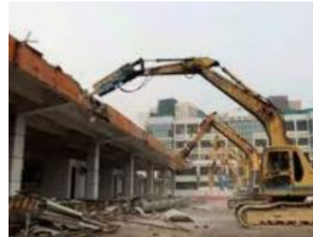
HEAVY MACHINERY ZONE
