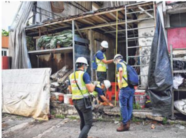
Officers from the Manpower Ministry's Occupational Safety and Health Division measuring a platform's height at a worksite safety inspection yesterday. The inspection was part of ramped-up enforcement efforts. ST PHOTO: FELINE LIM
