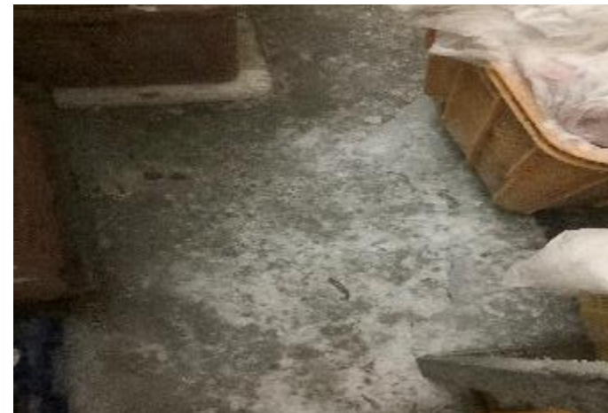
Ice on cold room surface
