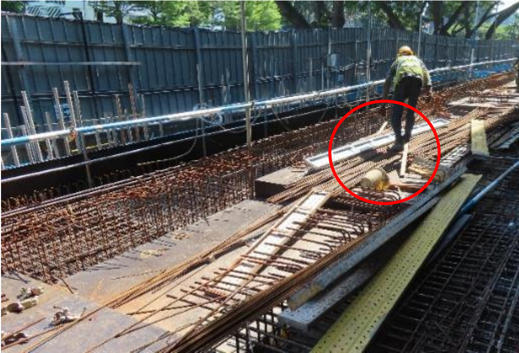
unstable work surface cluttered with rebar
