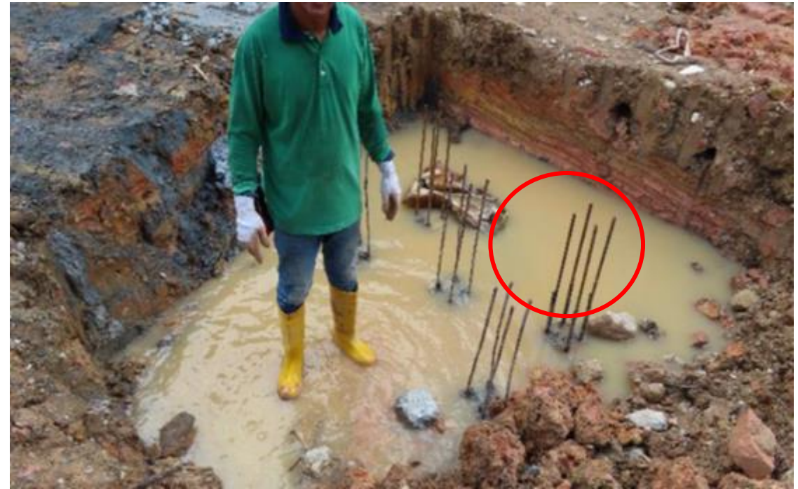
exposed sharp ends of rebars
