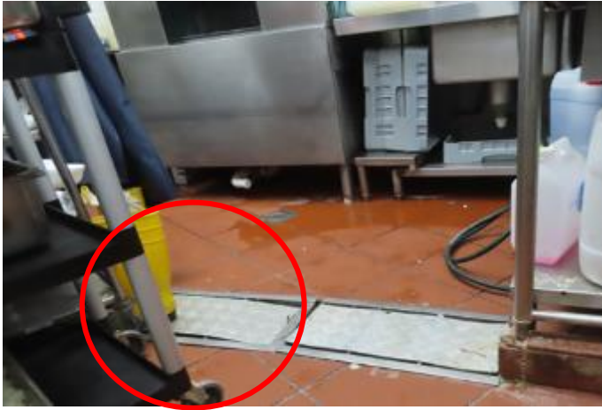
Sunken metal plate of drain cover
