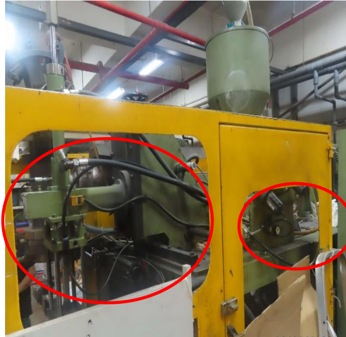
Missing guards/enclosure not replaced
