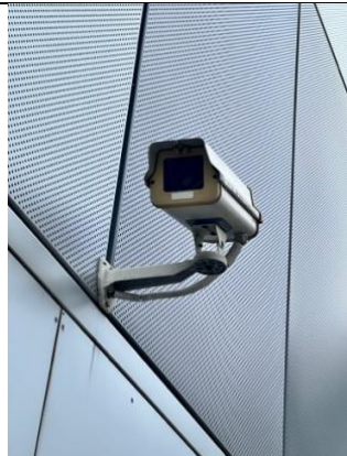
Figure 3: Bullet camera mounted on an exterior wall
