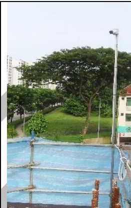
Figure 4: Bullet camera mounted on a specially erected support at a site under construction
