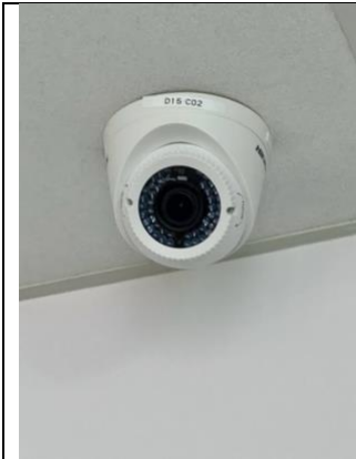
Figure 2: Dome camera mounted on an indoor ceiling
