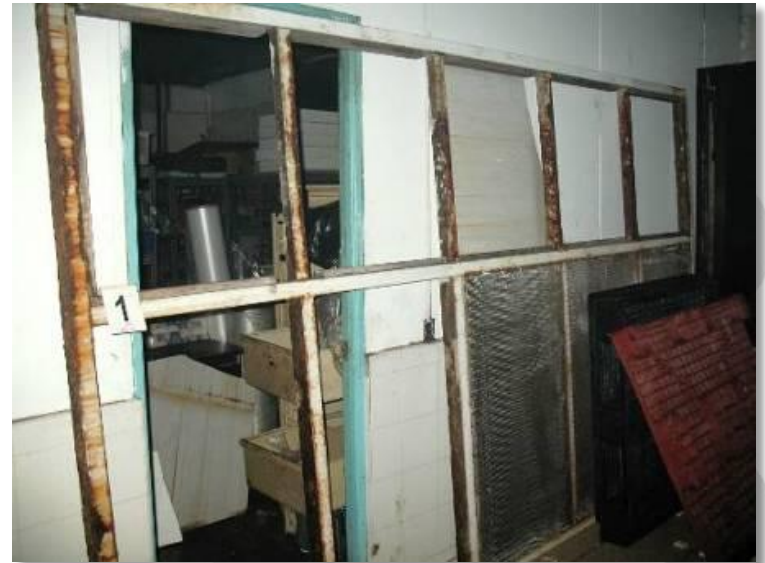
Figure 4a: Fallen window sash measuring 3.6 metres tall and 2.2 metres wide.
