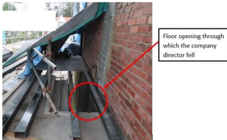
Overview of the accident scene.
